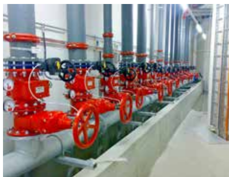
Installation sprinkler humide Source : JOMOS, Balsthal
