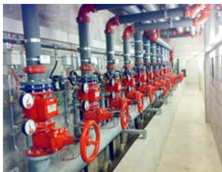
Installation sprinkler humide Source : JOMOS, Balsthal
